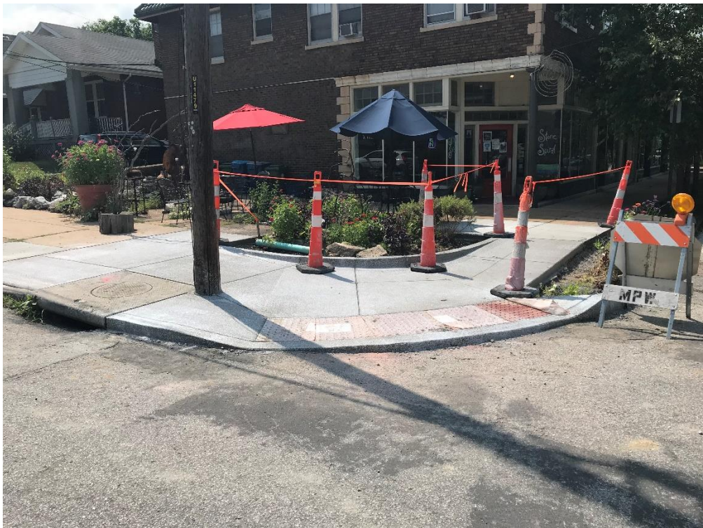
Handicap ramp at the SE corner of Lyndover Place and Sutton Blvd.
