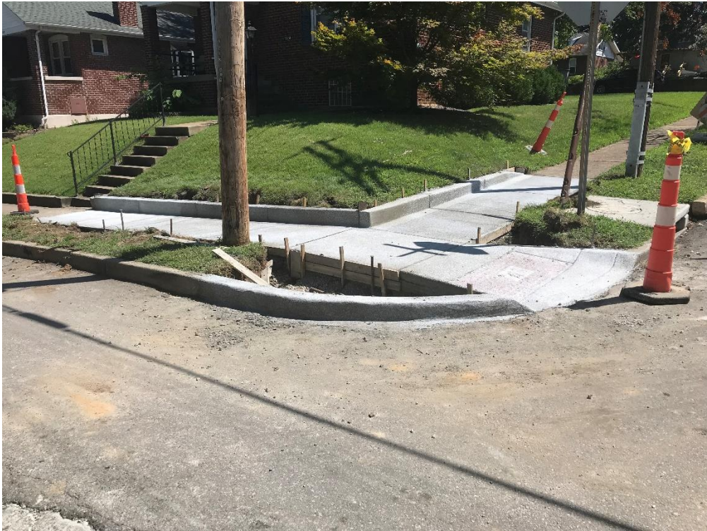
Handicap ramp at the SE corner of Richmond Place and Roseland Terrace.
